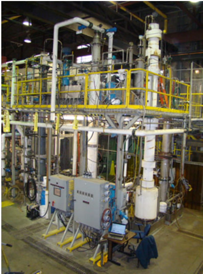
Figure 1: UNDEERC post-combustion CO 2 capture test facility
